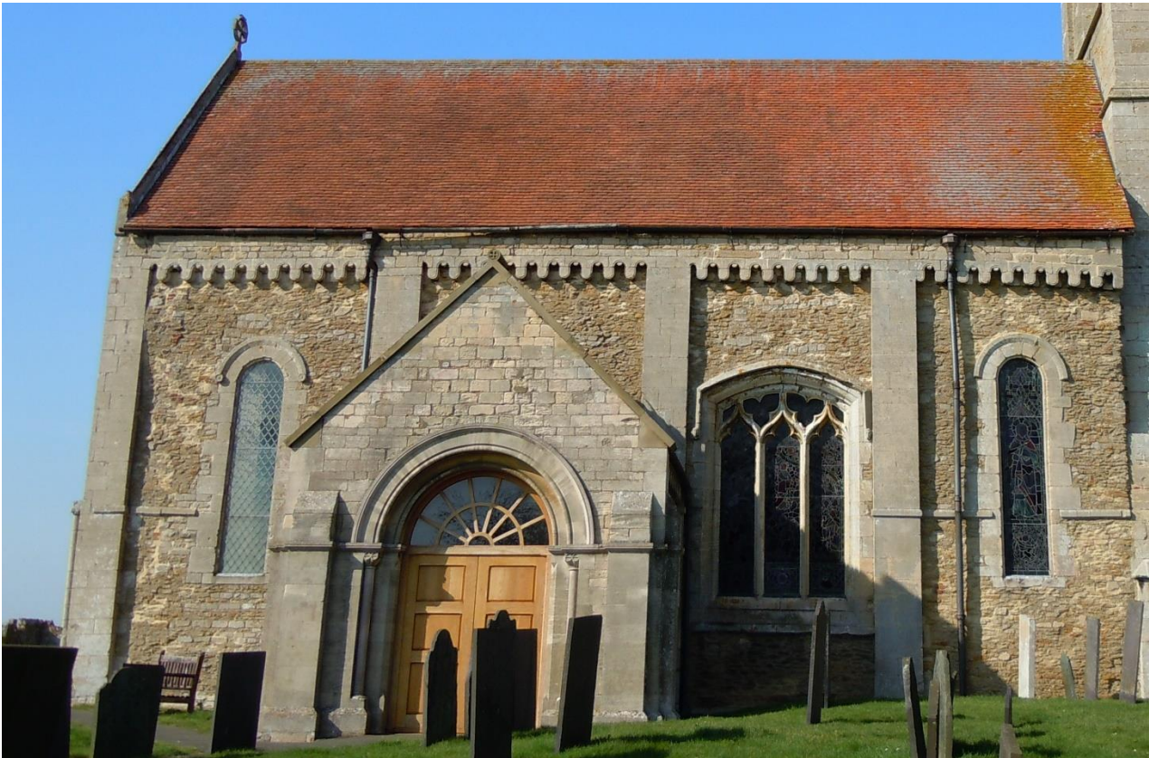
Above the south wall of the nave of Sempringham St Andrew showing the Norman exterior. The semi-circular lancet windows either end are of 1170s date as is the corbel table just below the roof eaves. The vertical sections dividing the wall up are known as pilasters and are an early form of buttress. The porch is 19 th century
