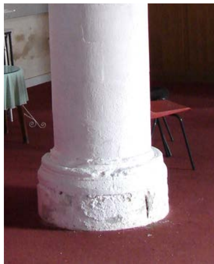
Note how the base of the column has salt damage and the wall beyond is growing mould - all because the moisture cannot escape through the carpet.
