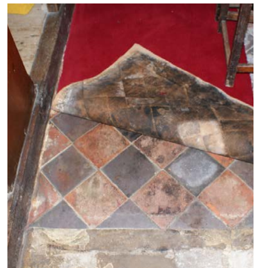
Black mould has grown because moisture has been trapped without adequate ventilation. Note too the beginnings of rot in the pew platform.
