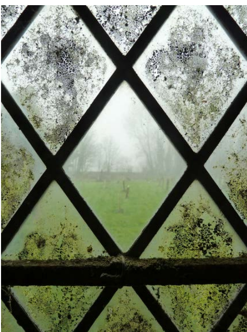
Fig. 6. Appleby, St. Bartholomew, plain leaded north window, no date. Internal loose dirt and accretions, centre pane being dry cleaned with a soft brush.
