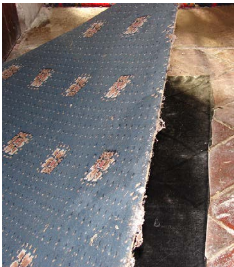
Impermeable plastic sheeting beneath a carpet is not to be recommended
